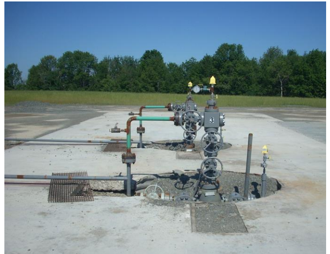
Figure 2: Shale gas production wells in Pennsylvania, USA. (Image from Wikimedia Commons)
